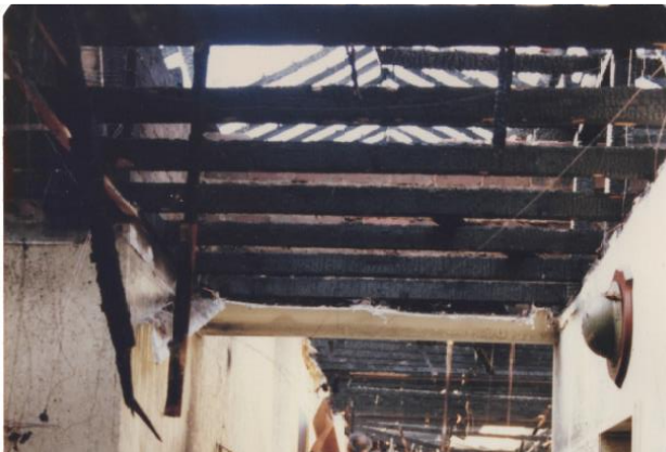
Another view of damage above the Main Hall
