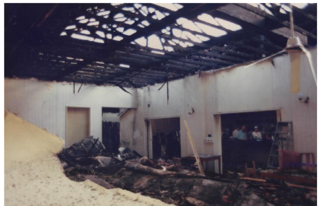
Damage to the roof above the Main Hall
