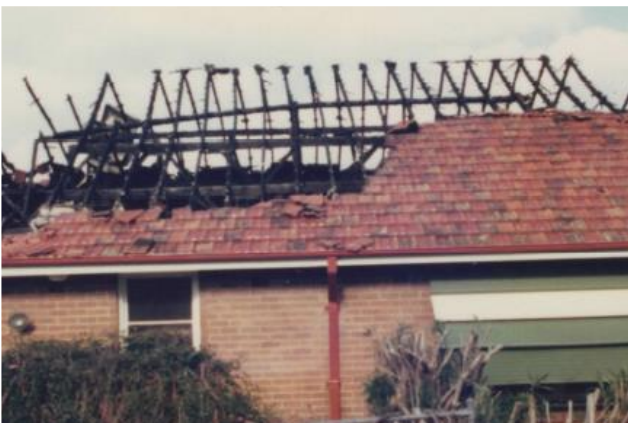
After the fire
